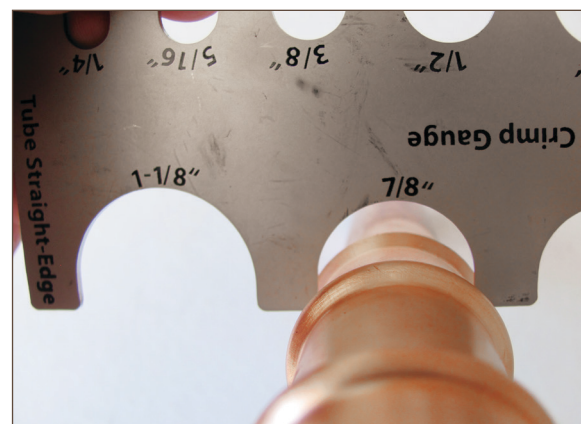
Figure 11.21. Un-crimped or improperly crimped fitting
