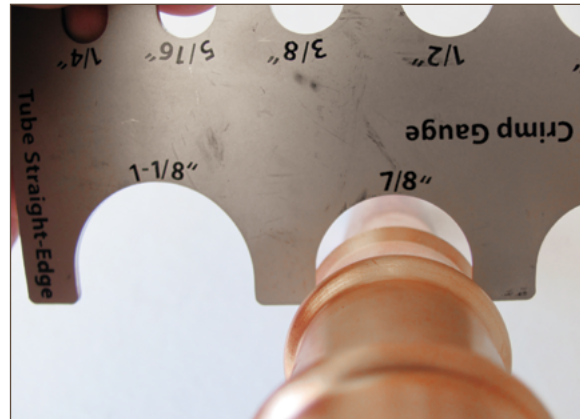
Figure 11.21. Un-crimped or improperly crimped fitting
